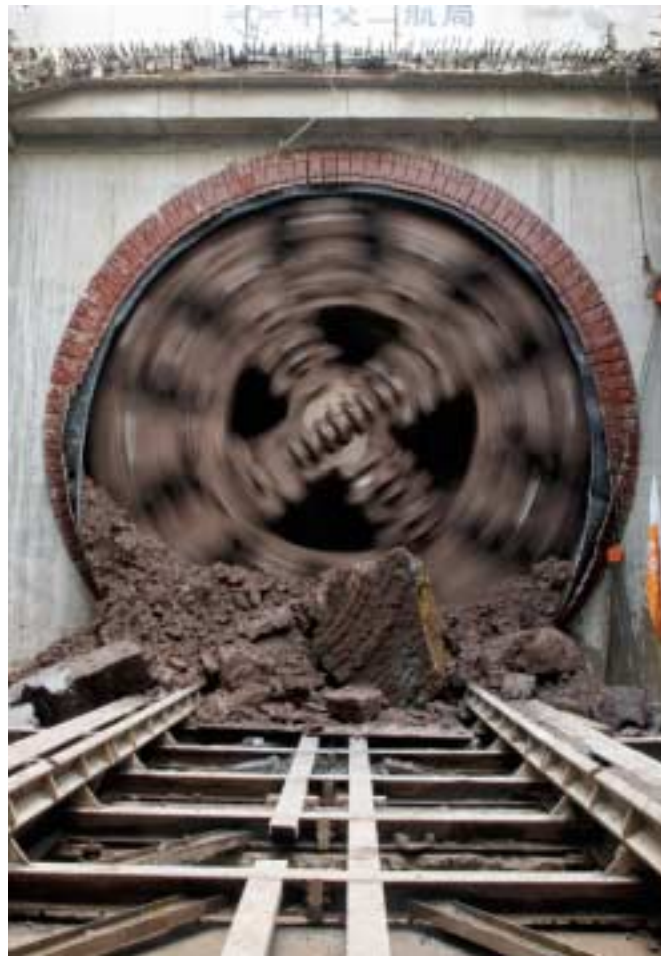
4 EPBs boring the Guangzhou Metro Project achieved 16 project records, along with rates of up to 377 m per month
