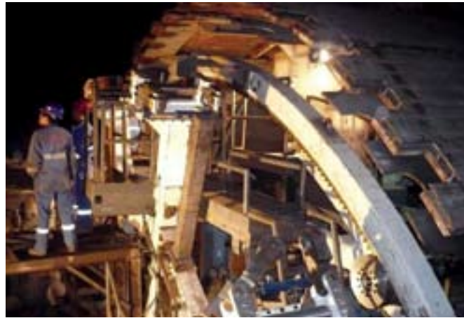
8 The McNally Support system was installed, consisting of a curved assembly of pockets on the roof shield, replacing the shield fingers on the Robbins Main Beam
