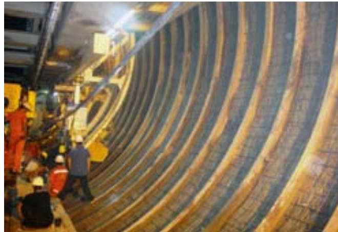
5 As of October 2010, the machines had advanced more than 1 km, and were excavating at rates of up to 595 m/month. Ground support consists of ring beams every 180 to 900 mm
