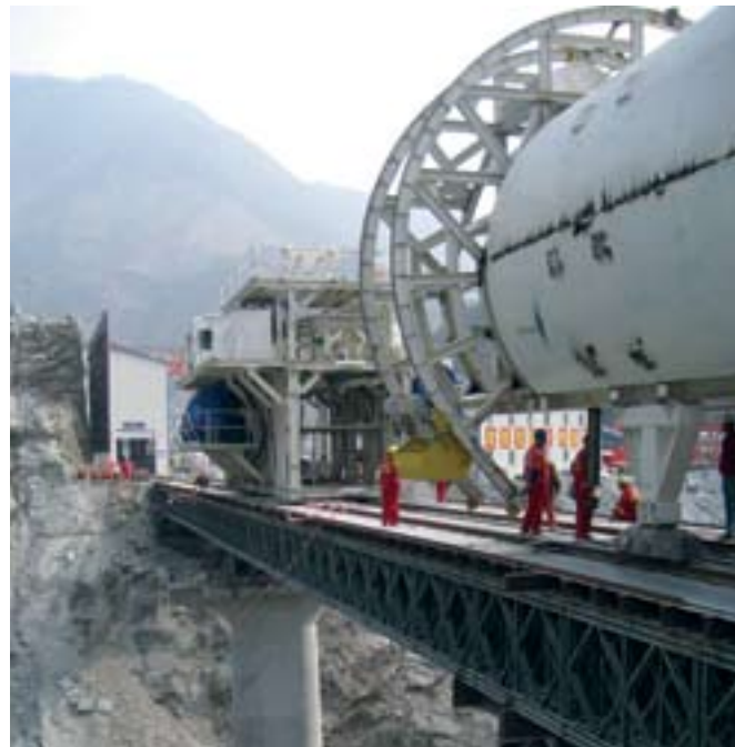
1 The two 10.2 m diameter Robbins TBM were assembled on bridges spanning a deep valley
