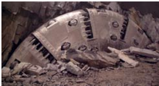
7 After severely unstable ground conditions were encountered, modifications were made to the Jinping-II TBM in a cross chamber
