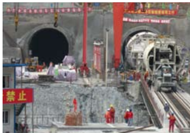
2 Both Robbins TBM for China's West Qinling Rail Tunnels were designed for high cover tunnelling without roof shield fingers
