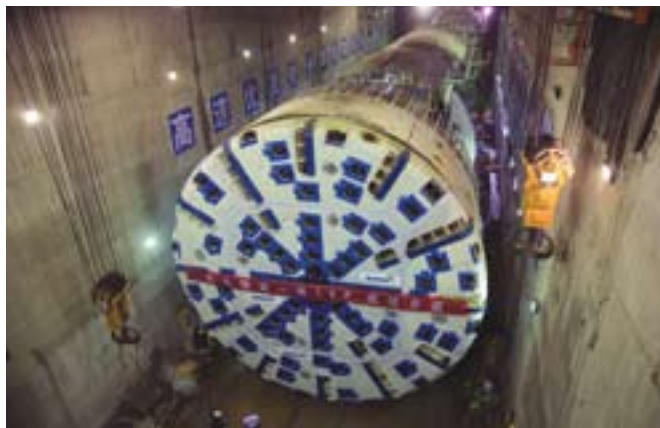
6 The 12.43 m diameter Robbins Main Beam at China's Jinping-II project was launched in October 2008
