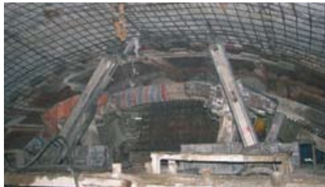
9 The Robbins 12.43 m Main Beam TBM at Jinping-II is currently excavating at rates of up to 128 m per week using a program of rock bolts and wire mesh
