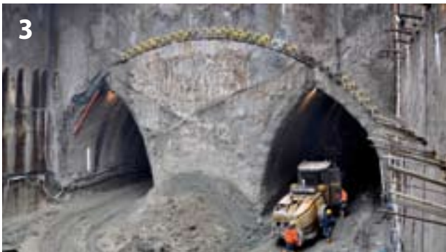
3 Ulmenstollen in der Baugrube Nord der U-Bahnstation 8-II Wall heading in construction pit north for the Metro Station 8-II
