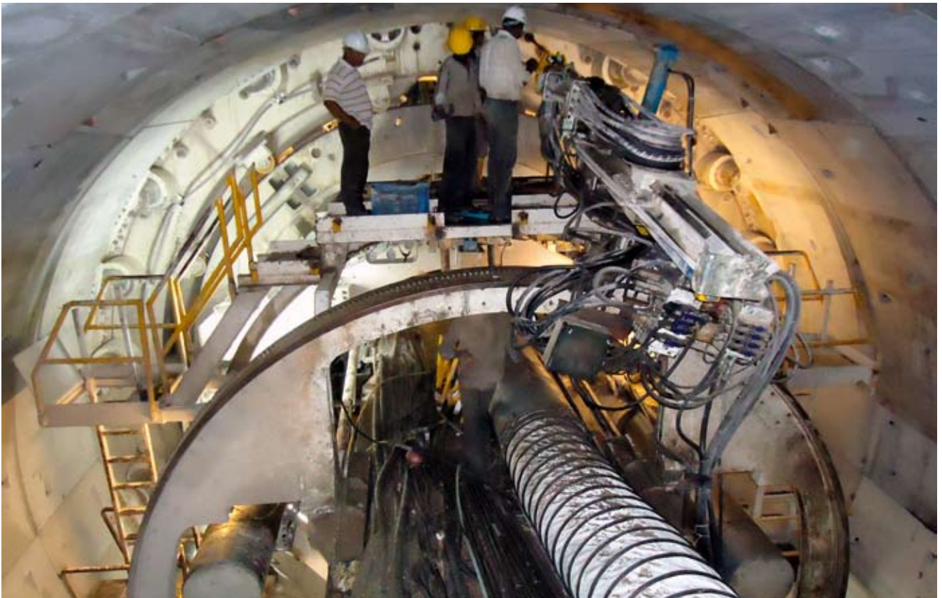
A strict program of probe drilling combined with primary and secondary grouting on the TBM has allowed the machine to advance through difficult sections of rock
