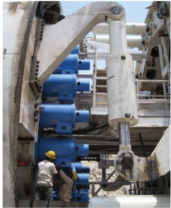
The international crew works daily in two 10-hour shifts plus a 4-hour maintenance shift, and consists of Robbins Field Service and locally trained labor
