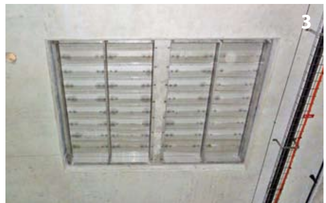
Fernsteuerbare Tunnelklappen Tunnel flaps operated by remote-control
