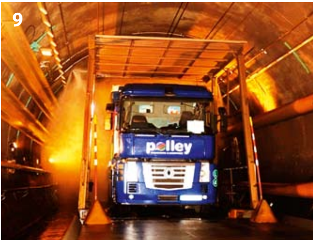
FFFS activation in the first SAFE station of the Eurotunnel
