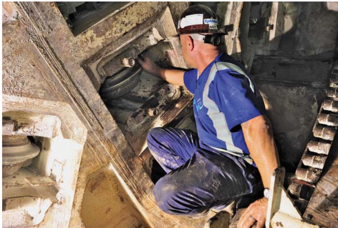
The remote cutter monitoring system, which enables continuous tracking of cutter wear, has been installed on 1 of the 3 TBMs
